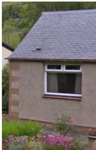
Detailing of adjacent dwelling – note mock quoins + dry dash render; minimal kick to base of roof + replacement slate roof with zinc ridge
